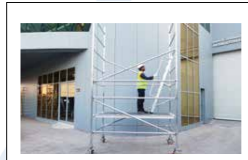
STEP -7 Place inclined ladder with handrail on the platform. Engage wind lock of stairway.
