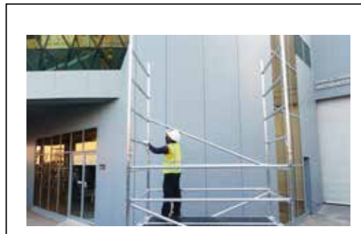
STEP-6 Fit diagonal brace from 3rd to 5th and 5th to 7th rung both the sides.
