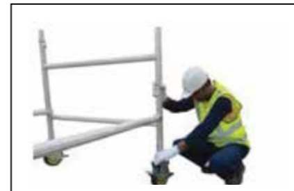
Step 4 Level the Mobile Tower . using spirit level. Use the adjustable jack of the wheel if require to level the tower
